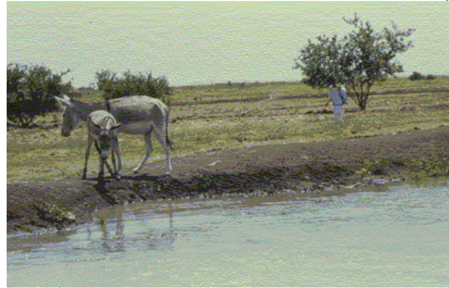
Canal side breakage due to animal burrowing
