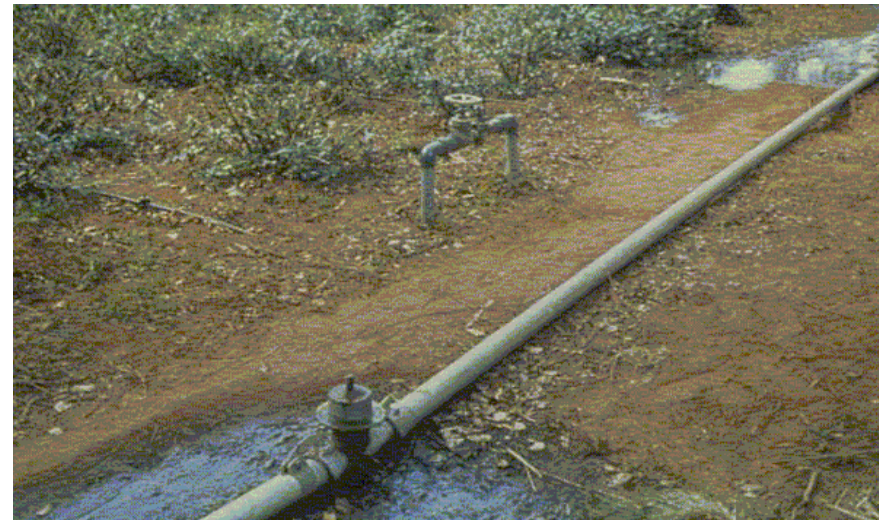
Leaking tubing for sprinkler irrigation
